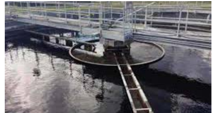
Figure #. South Regional Water Reclamation Plant
